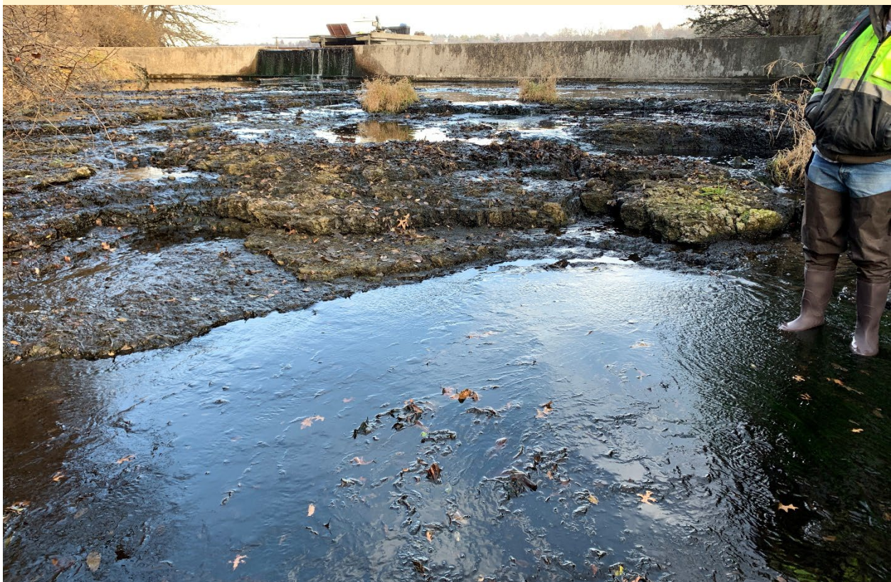
Photo: View rough rock surface of spillway channel and stop log weir
