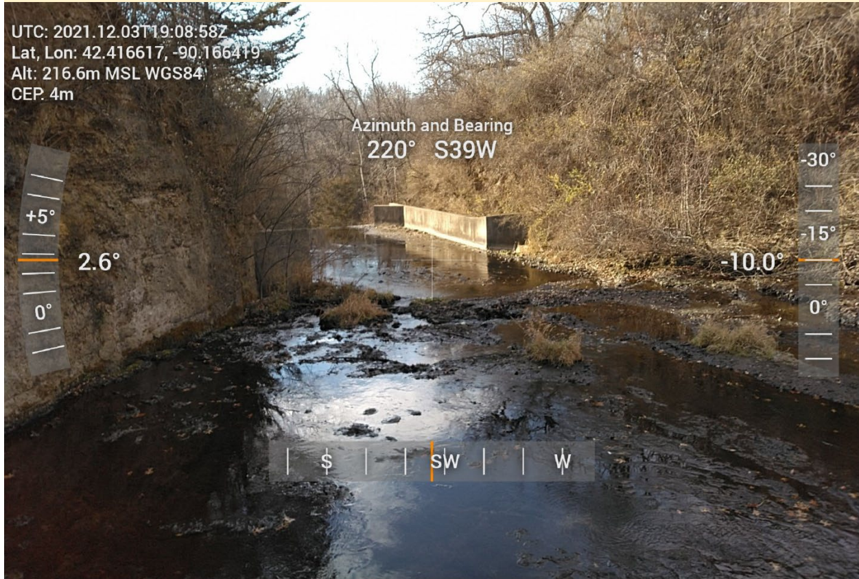
Photo: View of d/s channel of spillway showing rock base and existing training walls
