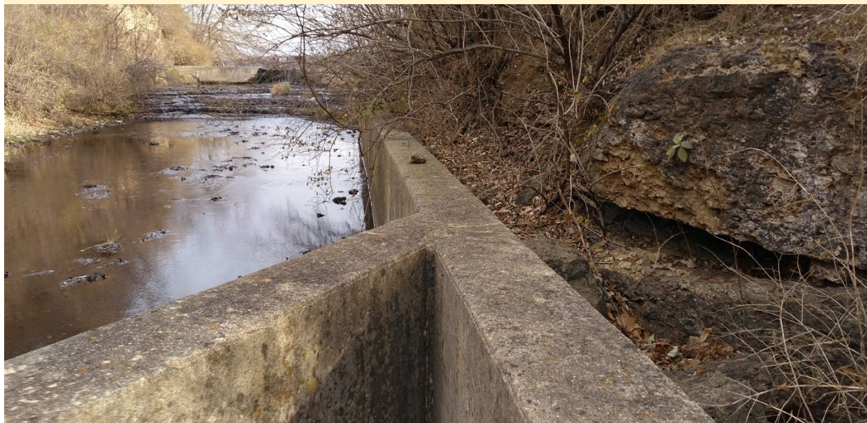
Photo: View looking NE along the SE training wall from the d/s end
