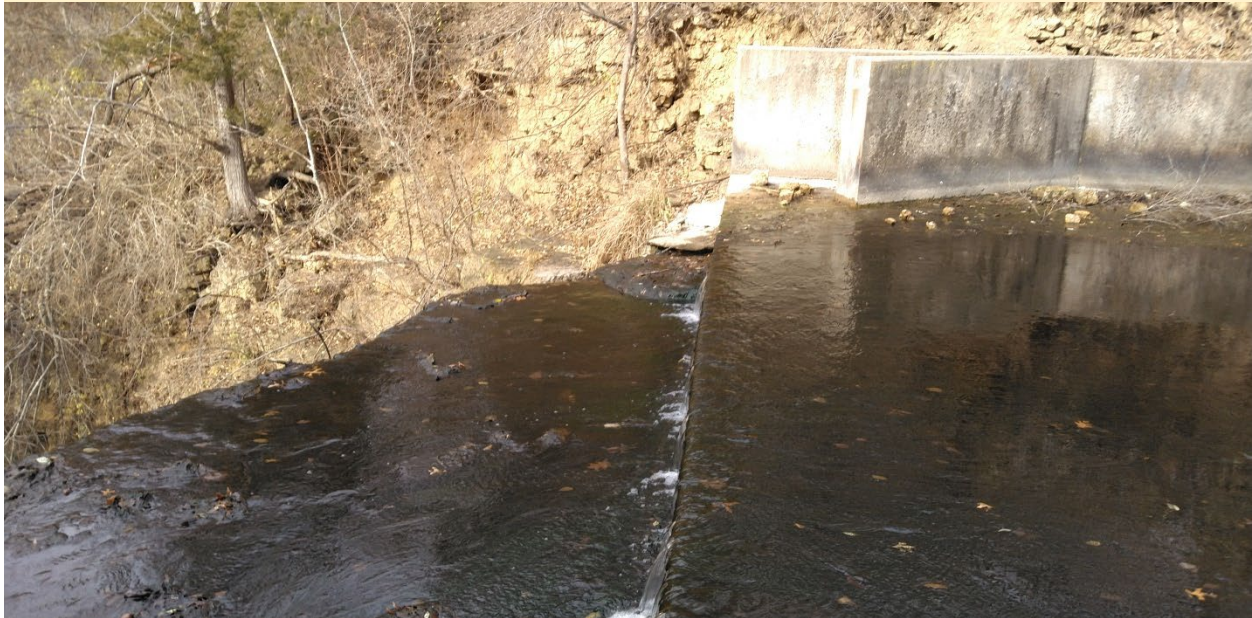
Photo: NW view of spillway discharge and overtopping erosion
