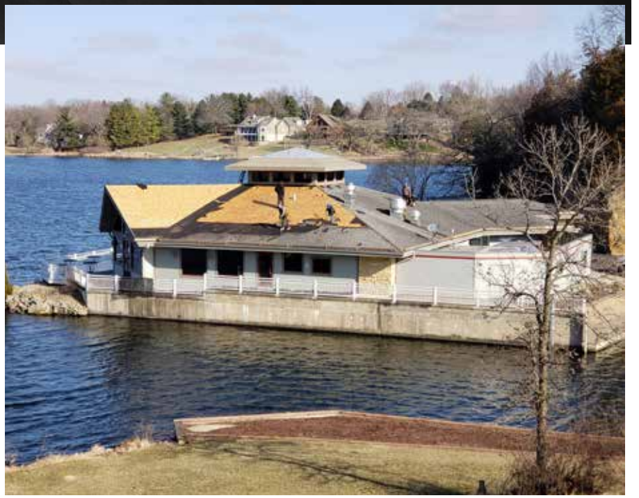
The crew from Strictly Shingles works hard stripping The Cove of its old roof.
