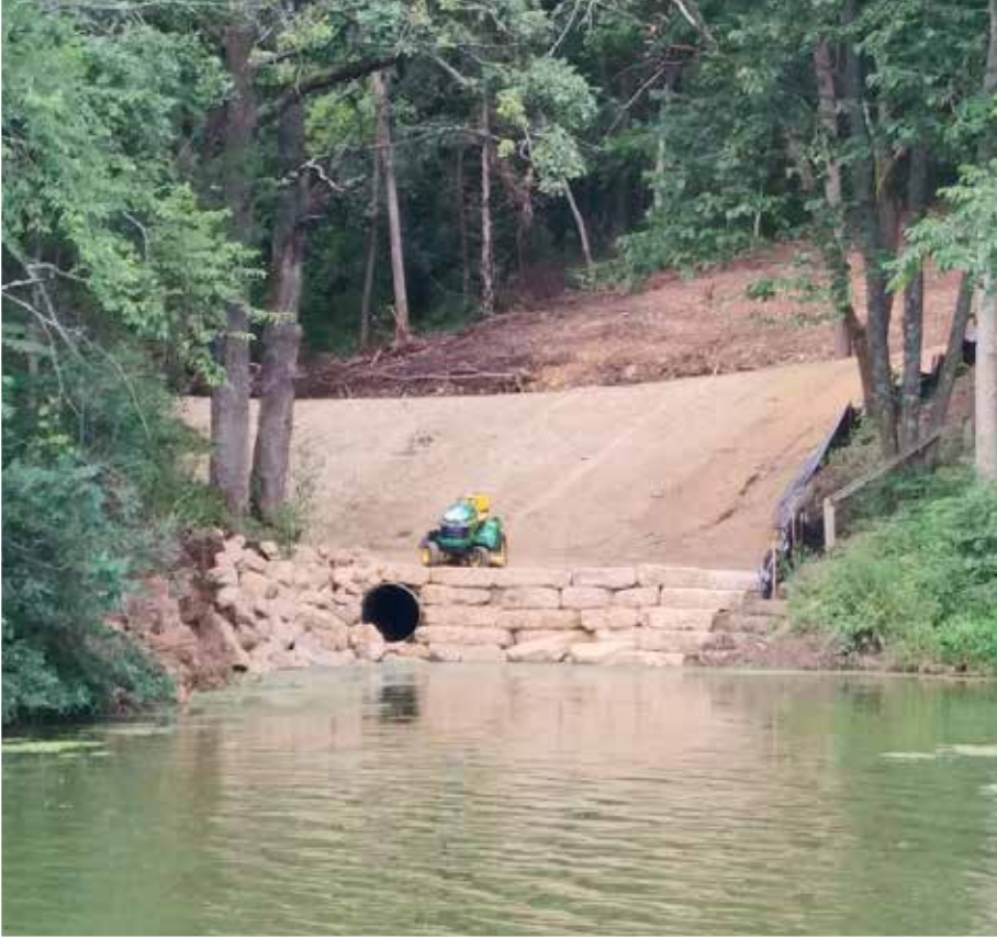
North Bay Dry Dam - This recently constructed dry dam in North Bay is part of the work done to mitigate flooding.
