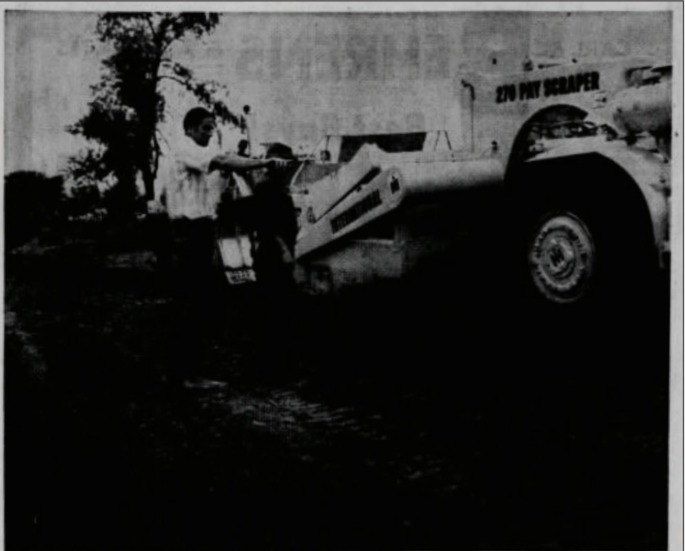
DAVE STORTZ, of the Braniger Organization's Apple Canyon Lake staff, points out grading area during construction
