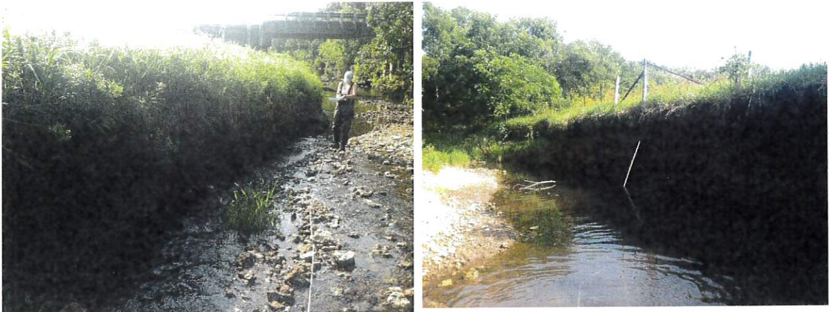
Figure 6-9. Downcutting and bank erosion in Stream Reach NB1
