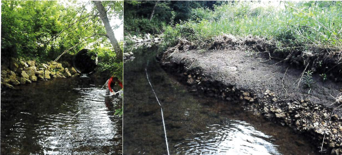
Figure 6-11. Erosion and bank condition in ID 1. Former bank is evident in these photos, however, spot treatment has not remedied larger issues.
